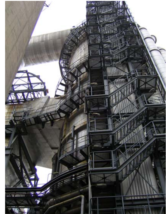
Desulfurisation, Yatagan thermal power plant
